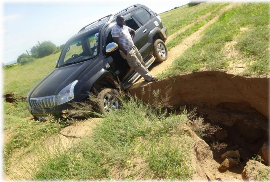
Figure 8: Peterlinus Ouma travelling in one of the deteriorated roads in the Ilemi Triangle
