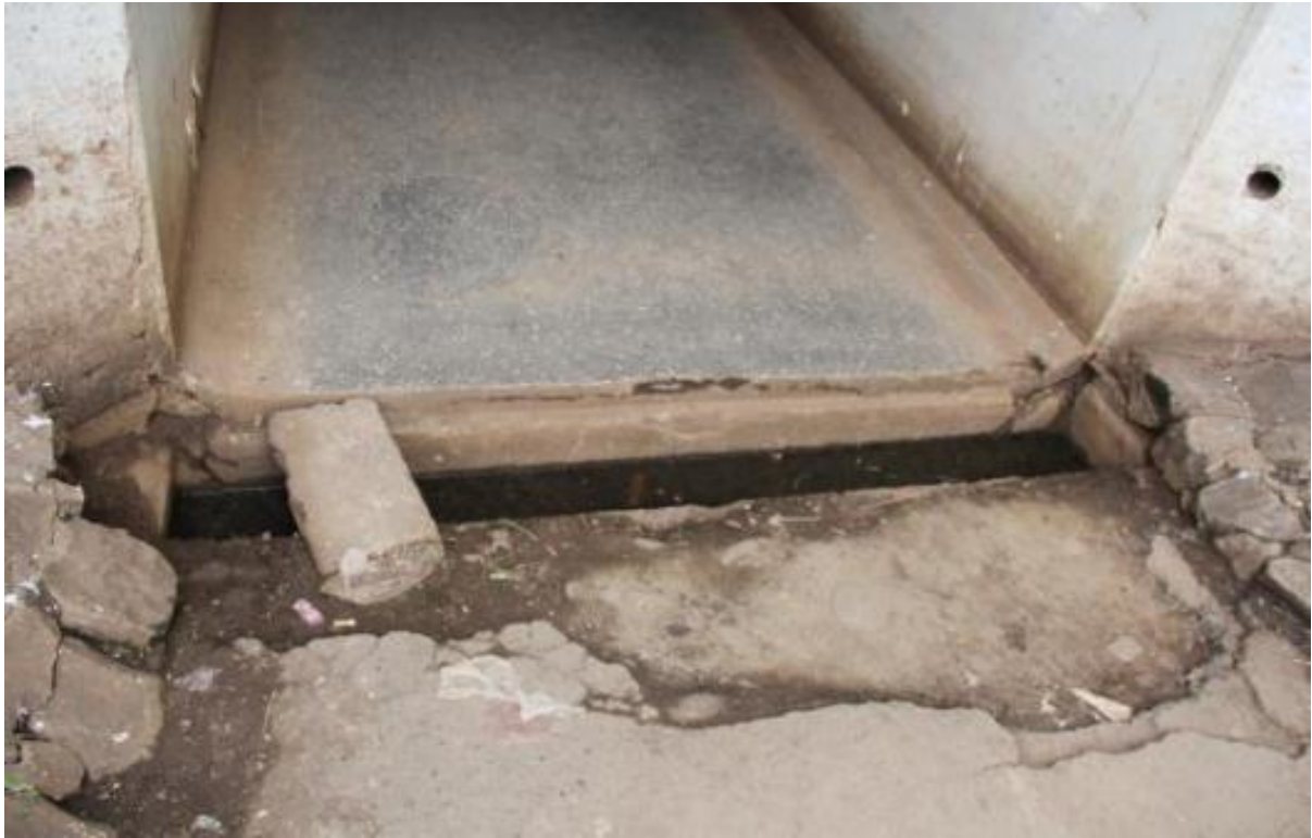
Plate 1-6: Open Drainage Sumps at the Entrances do not permit Universal Access and also poses safety threat to children, persons with disabilities and elderly pedestrians (Author, 2016)
