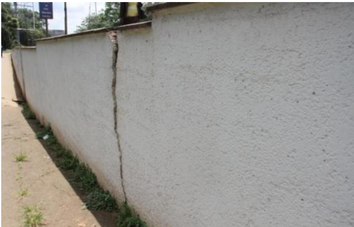
Plate 4-6: Cracks on the Retaining Wall Panels (Author, 2016)
