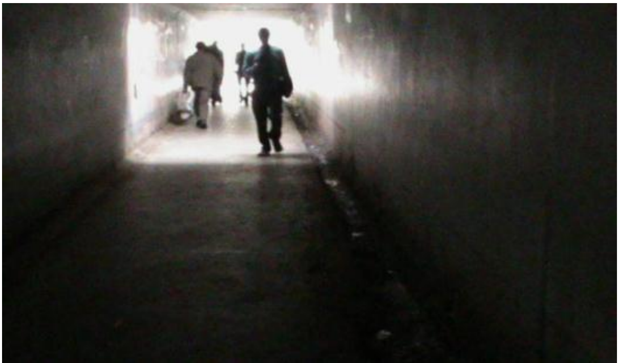
Plate 4-8: Light / Dark Contrast caused by Poor Lighting within the Tunnel
