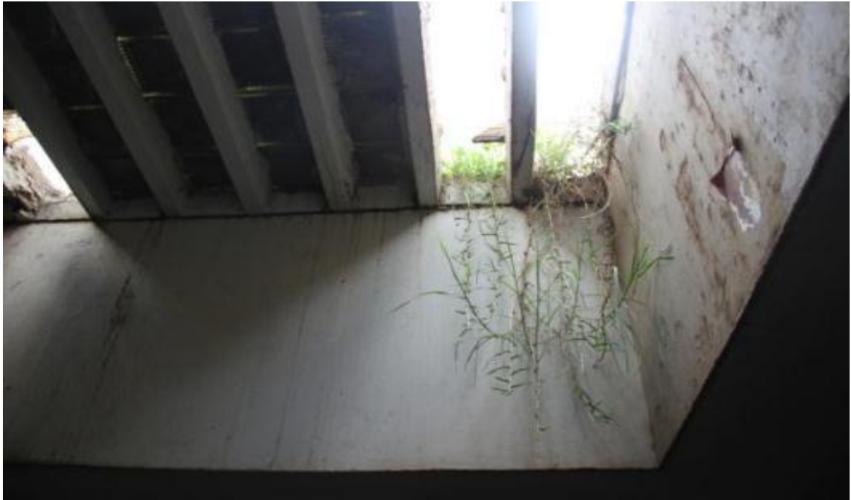
Plate 4-7: Damaged Skylight on the Tunnel Roof (Author, 2016)
