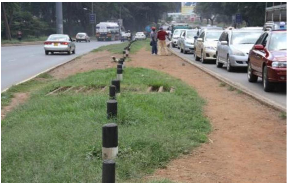
Plate 1-5: Absence of Pedestrian Channelization Barriers along the median encourages Jaywalking and Vehicle – Pedestrian Conflicts (Author, 2016)
