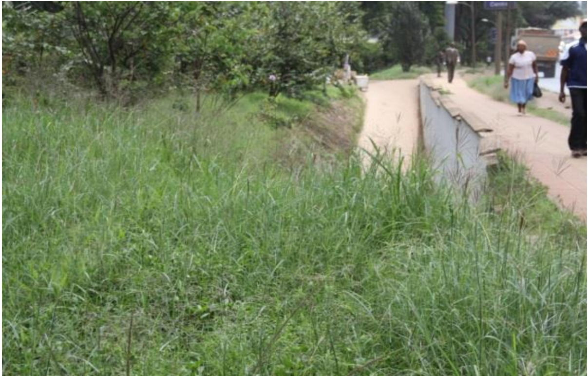
Plate 1-7: Overgrown Vegetation at the Tunnel Entrance (Author, 2015)
