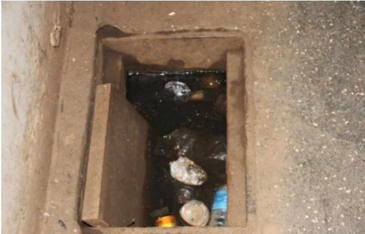
Plate 4-9: Filth inside a Manhole within the Tunnel (Author, 2016)
