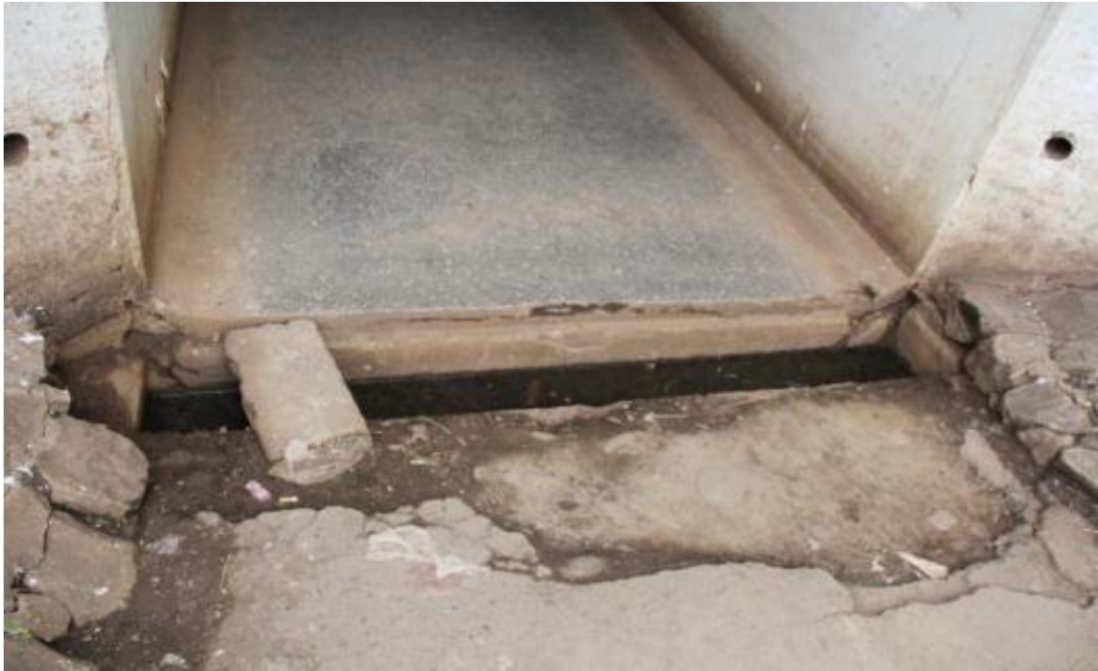
Plate 4-12: Condition of the Catch Basin at the Eastern Portal (Author, 2016)
