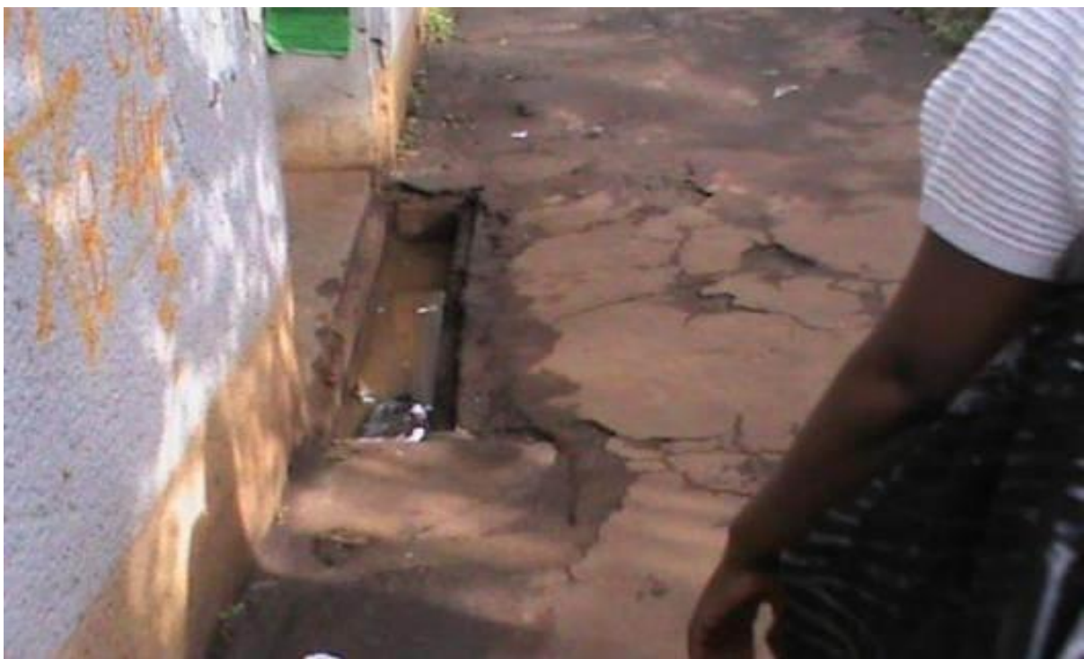
Plate 4-13: Condition of the Catch Basin at the Western Portal (Author, 2016)
