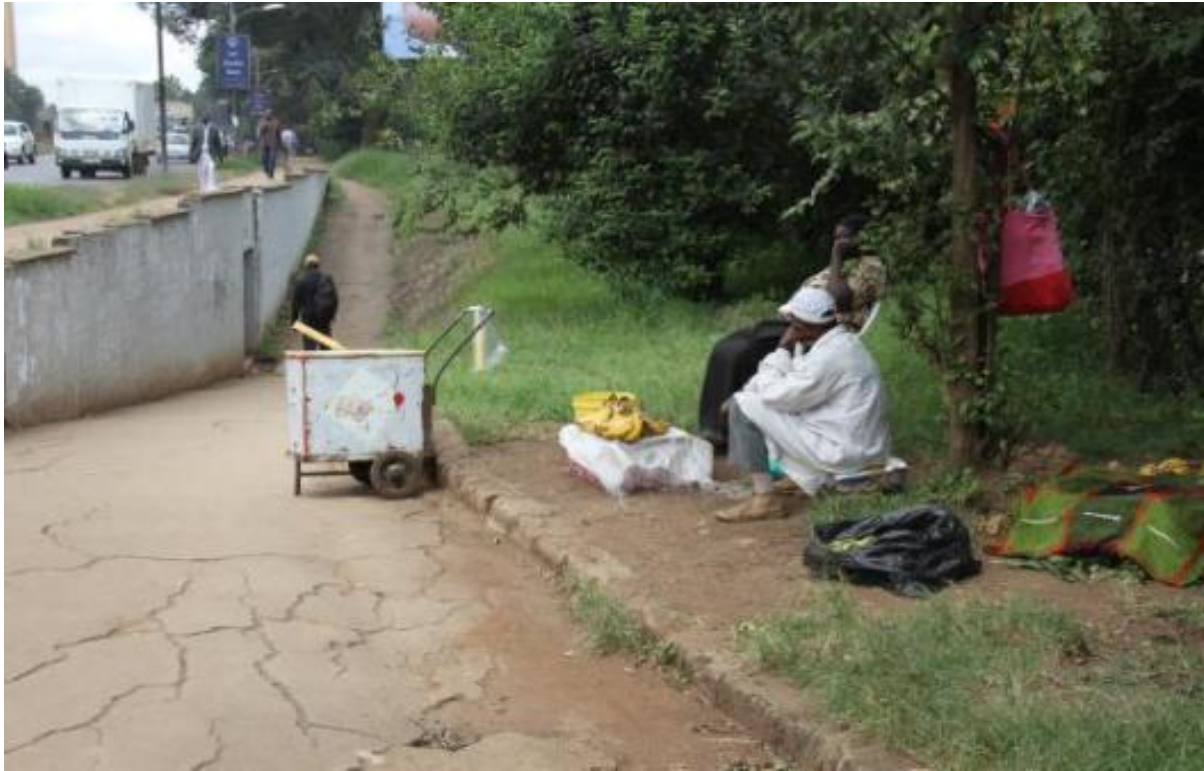
Plate 4-4: Ramp Type, Pavement Distresses (Cracks), and Static Activity (Vendor) on the Walkway (Author, 2016)
