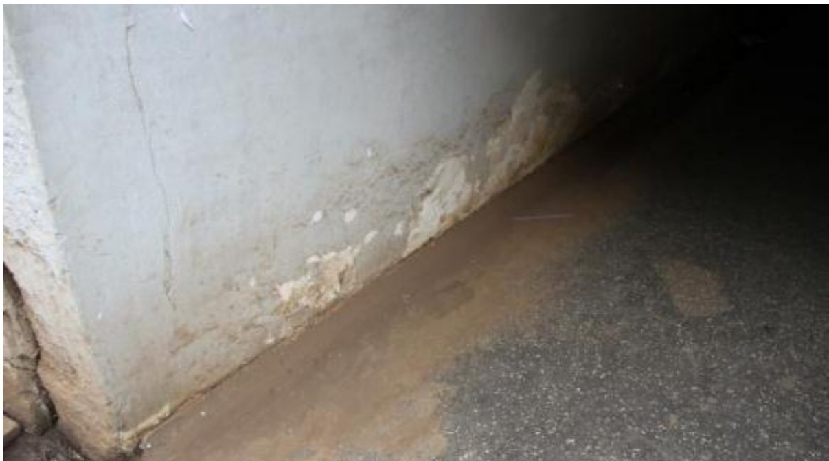
Plate 4-11: Flood Marks on the Tunnel Wall (Author, 2016)
