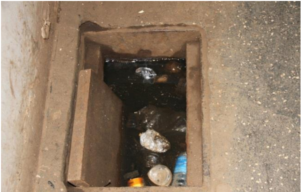
Plate 1-8: Open Filthy Drainage Sump at the Entrance (Author, 2015)
