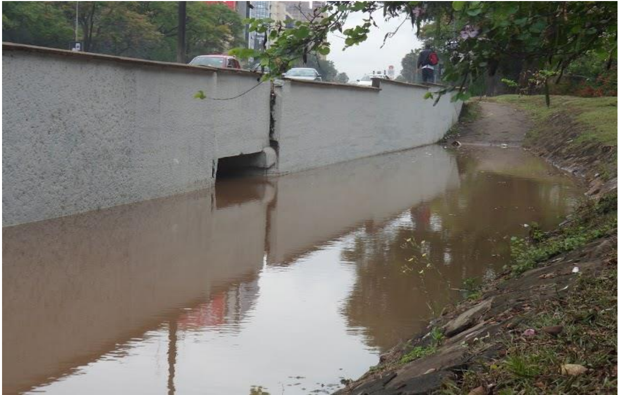
Plate 1-4: State of Drainage at the Eastern Portal when it rains (Author, 2016)
