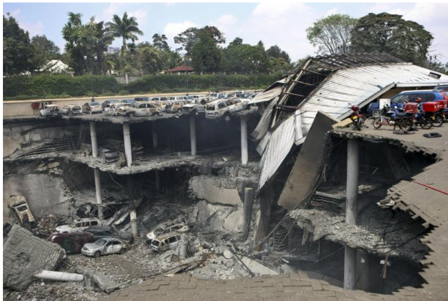
Figure 4: Exposed structural components of Westgate after terror attack
