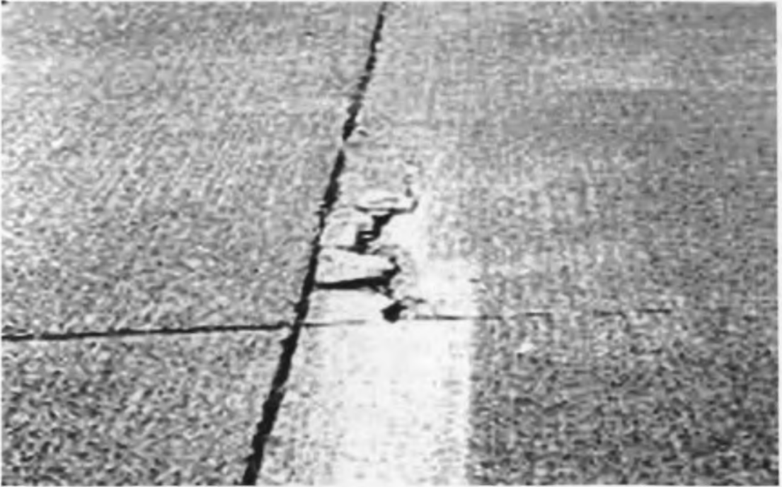
PLATE 02: A crack on a recently completed car park.
