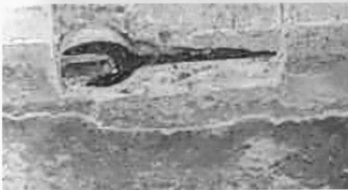
Plate 03: Poor Workmanship allowed this spanner to be dropped into the shuttering before the concrete was poured. The spanner has rusted causing the surface to spall.
