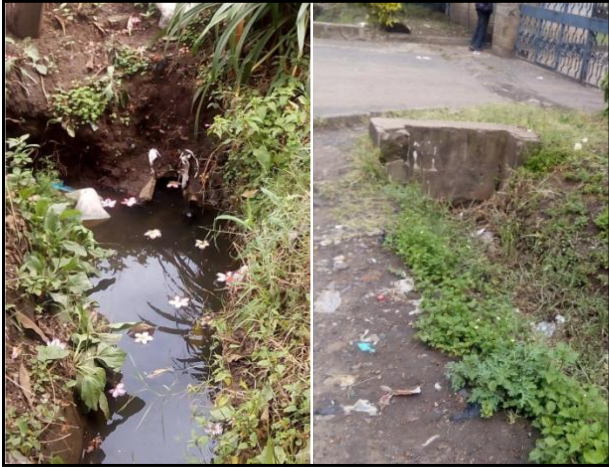
Plate 4-3: clogged drainage systems
