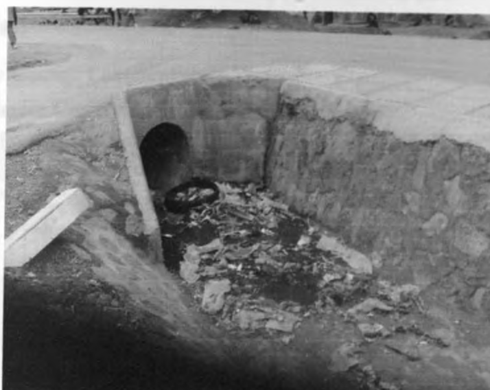
Figure 4.27 Waste dumping in Storm Drains
