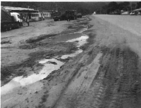
Figure 5.8 Stagnated water due to lack of storm Drains on part of the Maai Mahiu – Naivasha Rd.
