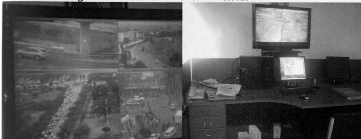
Photo 2: Monitoring Cameras at Nairobi Area Control Room
