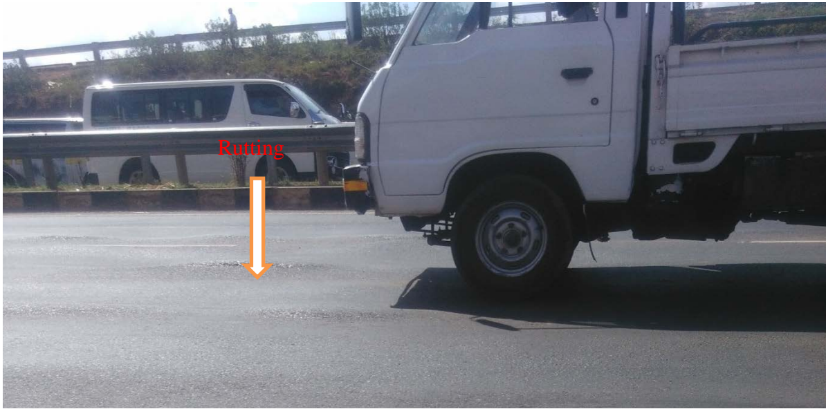
Figure 1.4 Rutting LHS pavement (at km 20+000 from Kenyatta University to Thika) (Source: Author, 2016)
