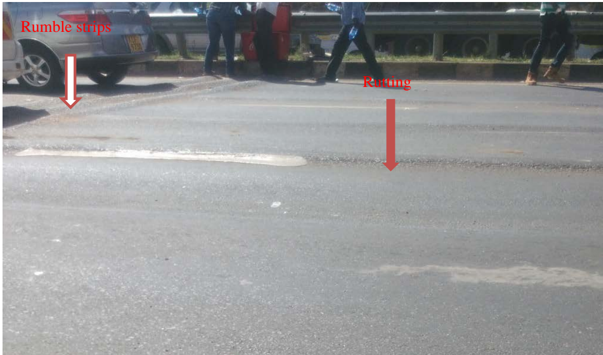
Figure 1.2: Rutting of LHS pavement (near the speed bumps at km 11+000 from Kenyatta University to Thika) (Source: Author, 2016)
