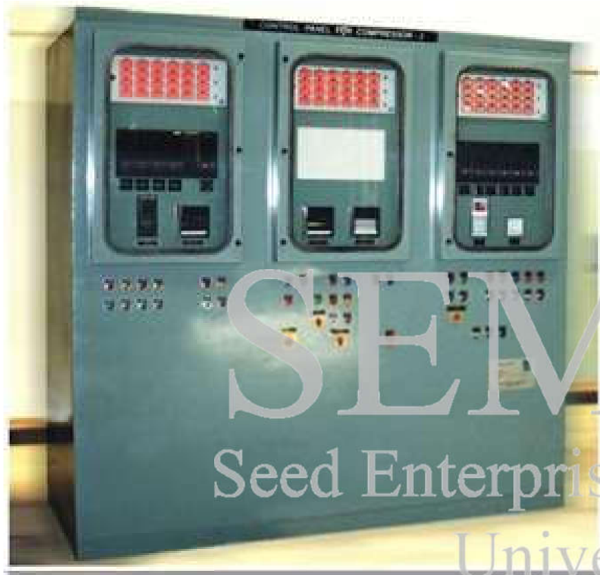
Control panel used in the processing plant
