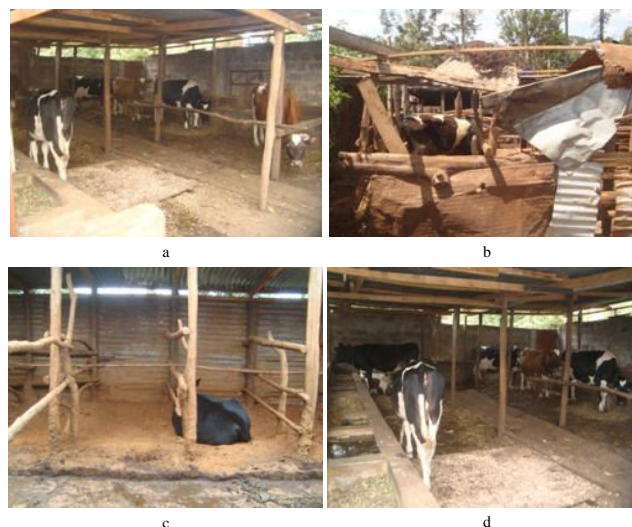
Photo 4: State of iron sheet roofing and walling system in the farms evaluated for welfare of dairy cattle in the smallholder production systems in Nairobi and its environs (July 2009 – October 2009). a- Complete iron sheet roofing (curved arrow), b- collapsed iron sheet roofing (straight arrow) c- walls made of ironsheet and d -walls made of concrete.
