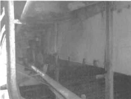
Photograph 4.7 Axial fan and steam pipe with nozzles for moisture correction
