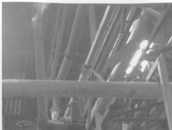
Photograph 4.5 A leaking safety valve
