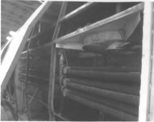
Photograph 4.6 Radiators and axial fans in drier
