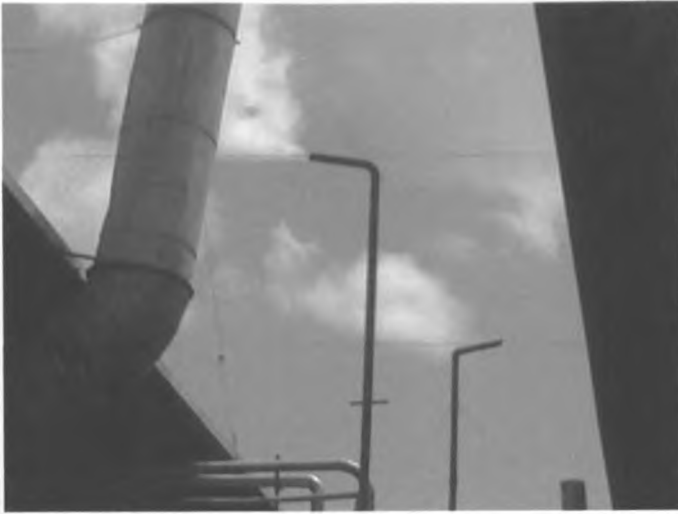
Photograph 4.11 High pressure flash steam from condensate pumps
