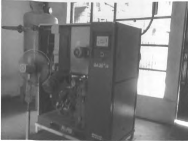
Photograph 4.15 Compressor 1 with inbuilt air dryer NB: external fan cooling the unit.
