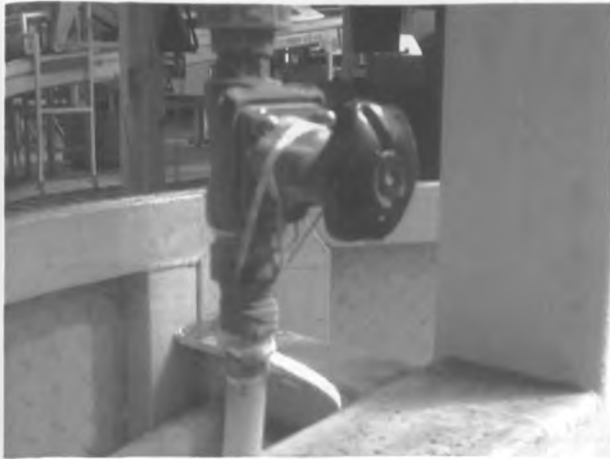
Photograph 4.16 Poorly fitted air hose
