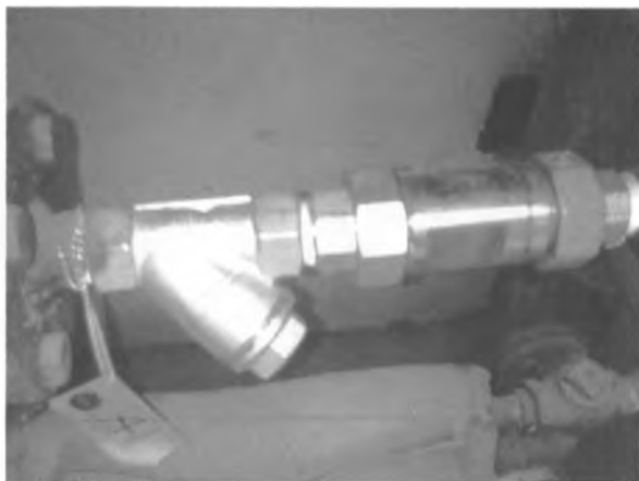
Photograph 4.8 Orifice steam trap
