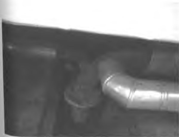
Photograph 4.10 Un-lagged condensate pipes in underground drain channel
