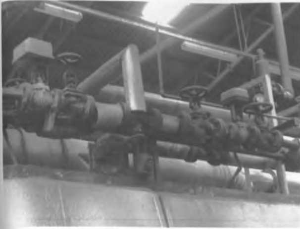
Photograph 4.3 Poorly lagged valves
