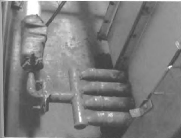
Photograph 4.4 Poor lagging line 2 cylinders (group trapping a poor practice)
