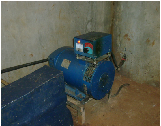
Fig. 49 the Turbine and Generator
