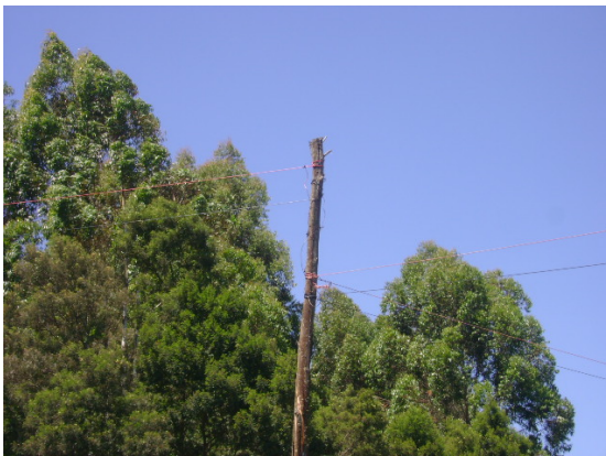
Fig. 40 power Distribution System
