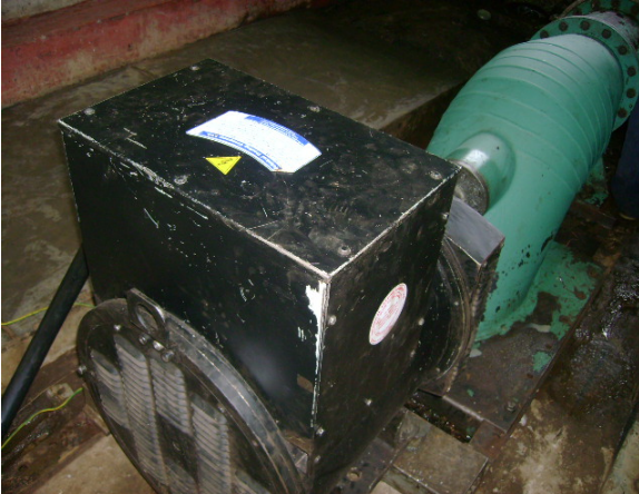
Fig. 23 the turbine and Generator
