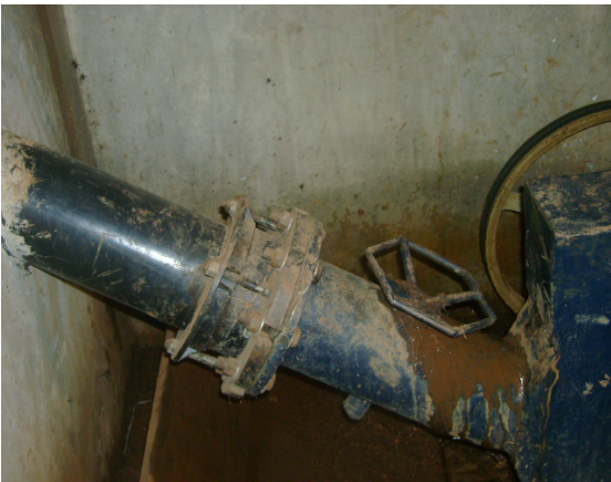
Fig. 48 Penstock termination to Turbine
