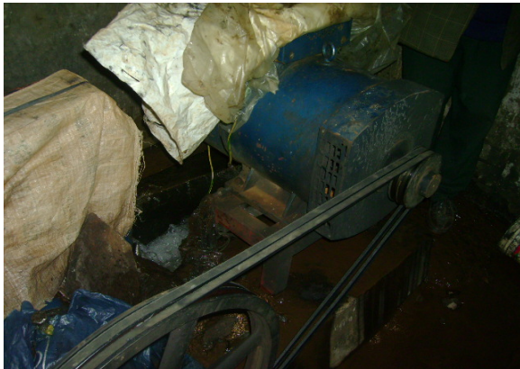
Fig. 37 the turbine system
