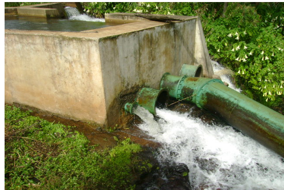
Fig. 20 outlet to the penstock
