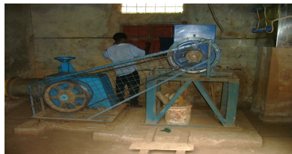
Fig. 4 The generating Equipment
