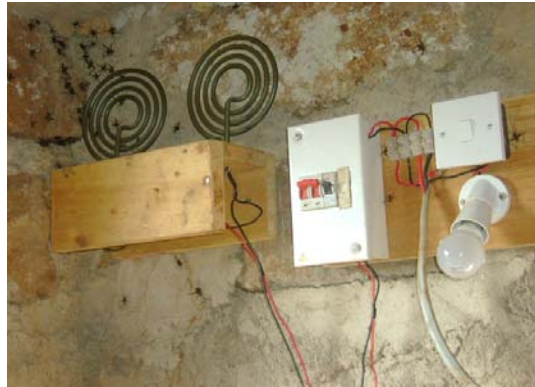
Fig. 51 electric coils for power dumping
