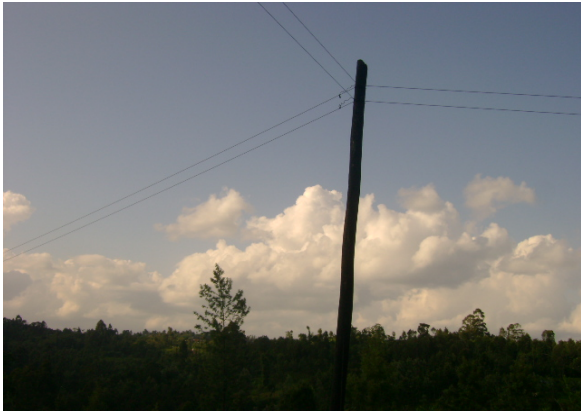
Fig. 52 power distribution system
