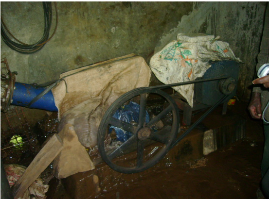
Fig. 36 inside the Powerhouse
