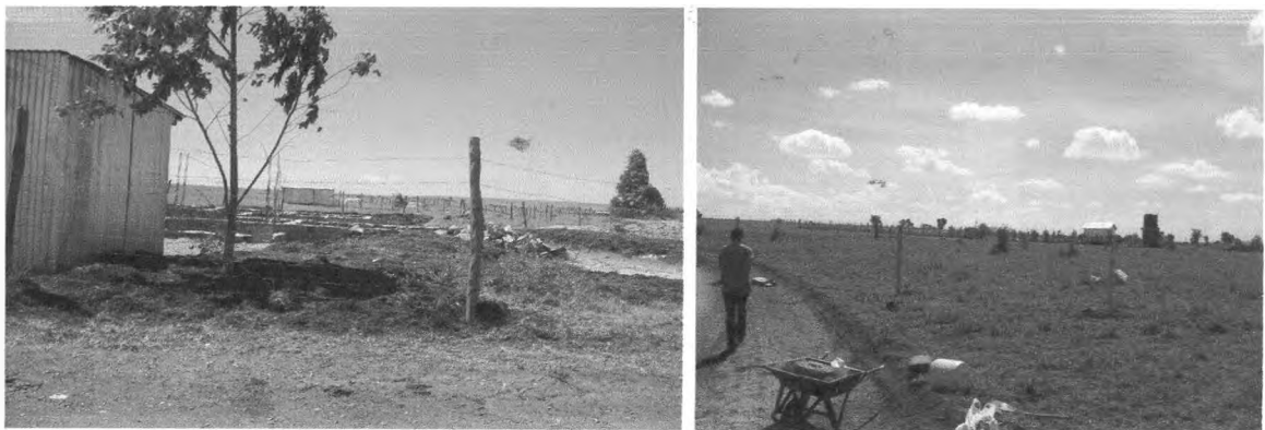
Figure 13: Newly subdivided plots under construction (Left) and fencing in progress (Right). Source: Field survey,2008.
