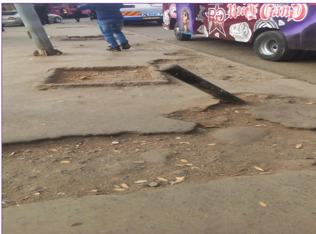
Plate 2: Poor Condition of the Pavements
