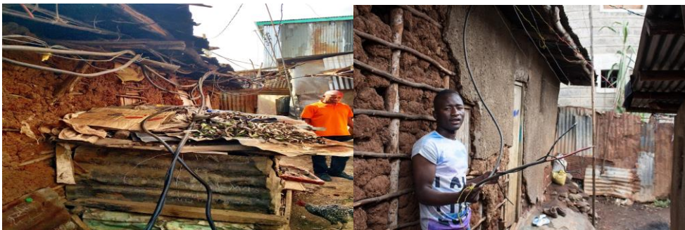
Plate 9: Substandard wiring in the slums
