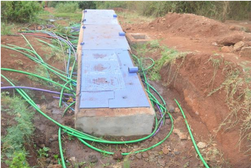
Plate 8: Water Meters Chamber
