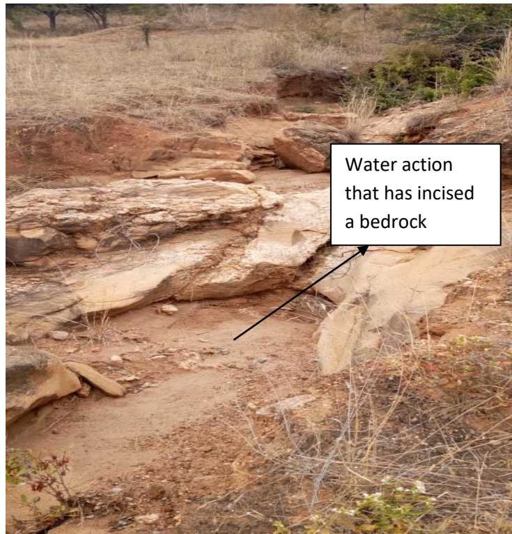
Plate 5.10: Water action along the backslope
