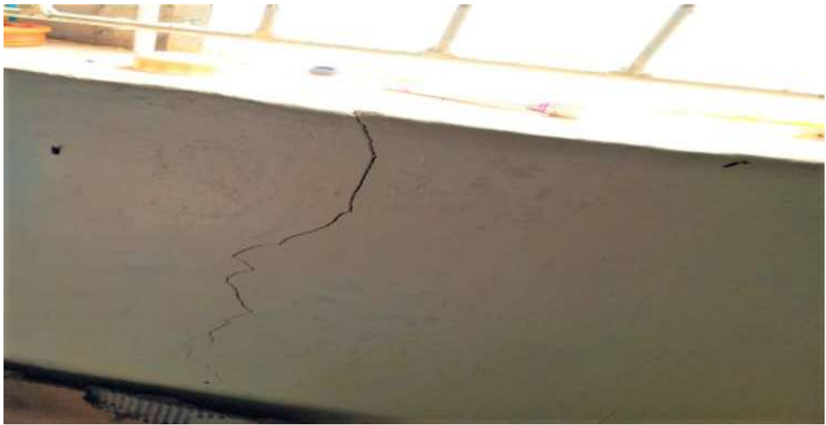
Cracks in the houses of residents
