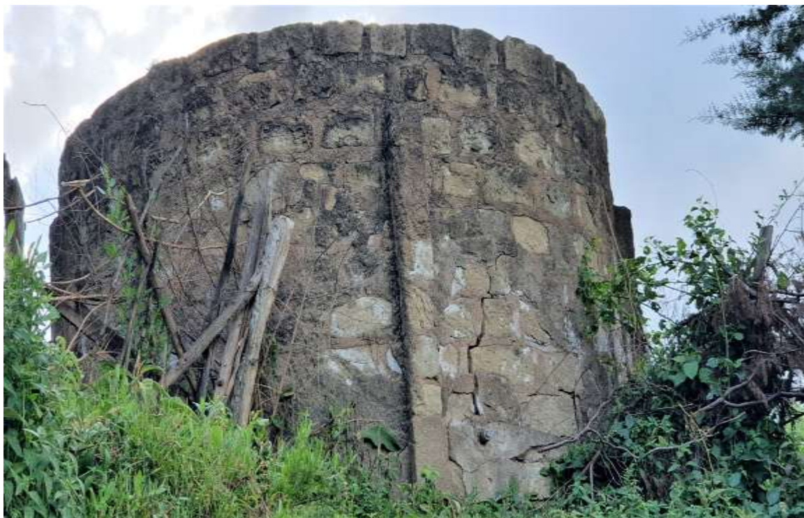
Cracked tank due to blasting and quarrying activities near it
