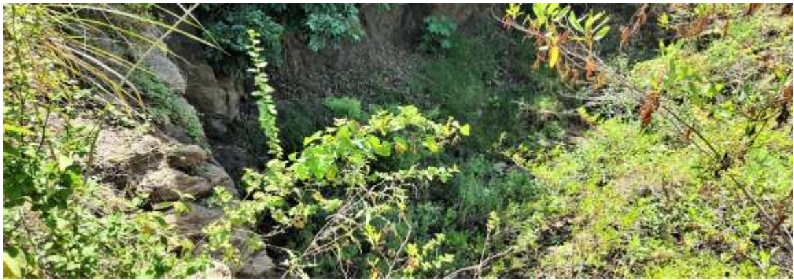
Uncovered pit by the road side endangering the lives of residents and livestock
