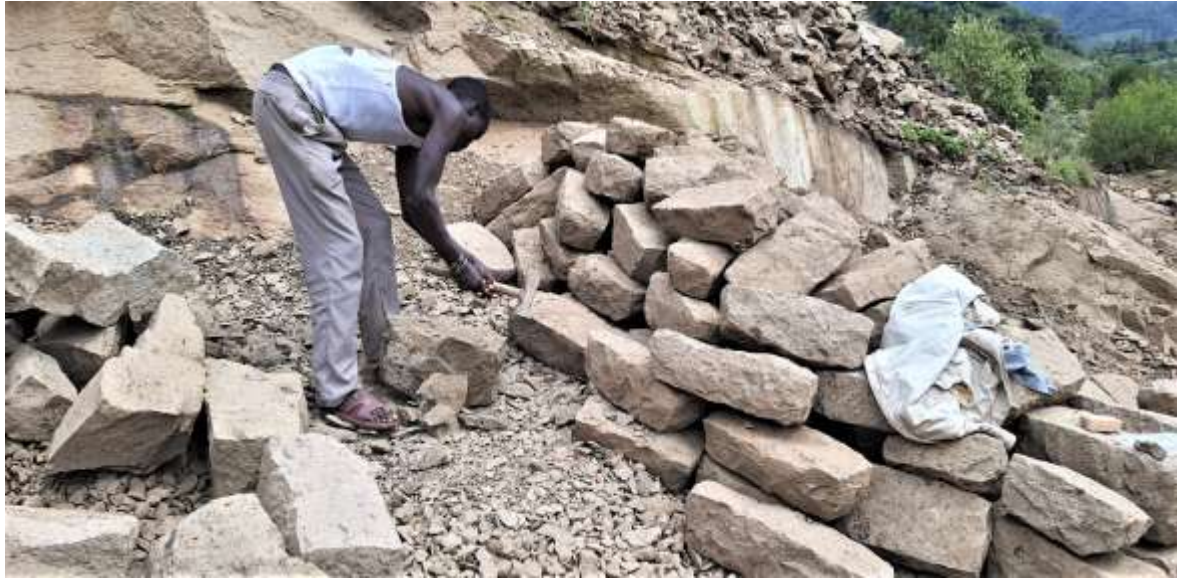
Quarry worker going about his daily activities without protective gear
