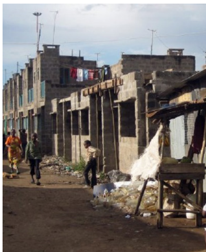
FIGURE 10 Implemented and occupied houses in the background, ongoing construction and a shack in the foreground Source: Author 2005
