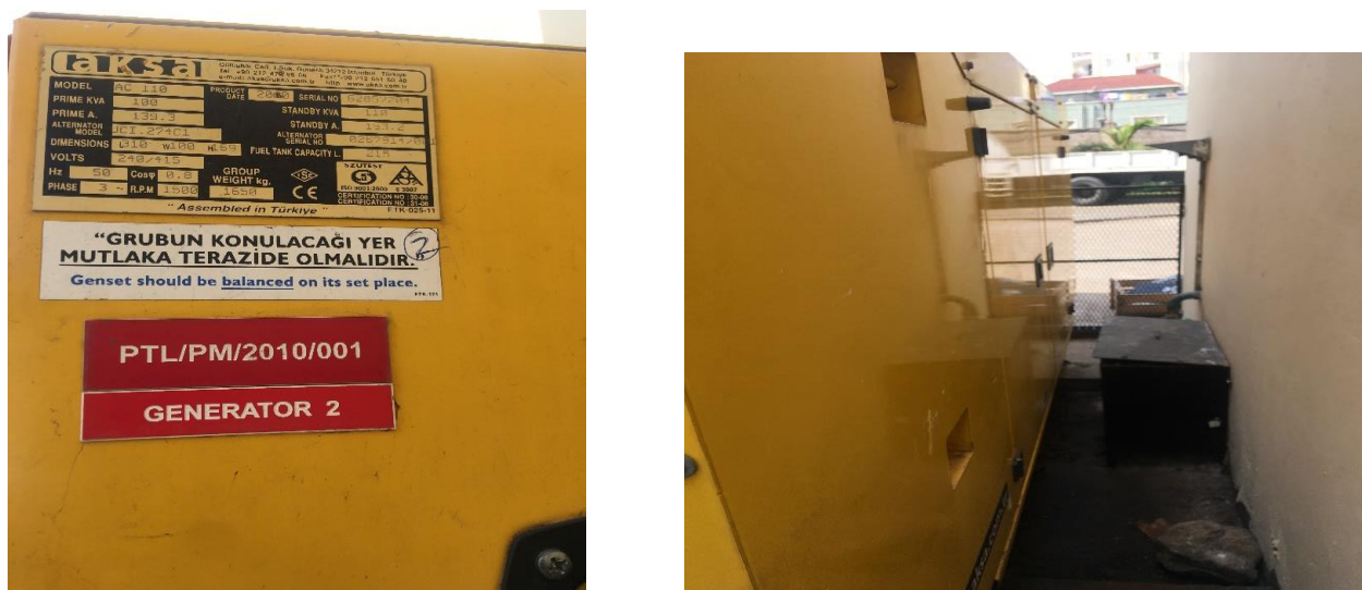
Figure 3.3: 100KVA Backup Generator
