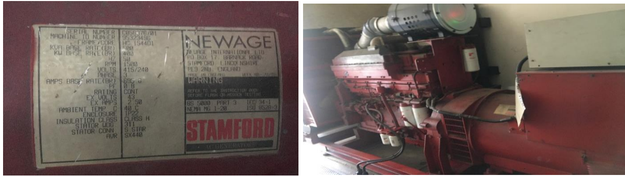
Figure 3.4: 500KVA Backup Generator
