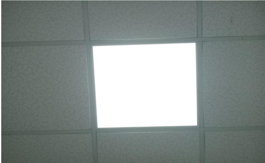
Figure 4.7: Existing Ceiling LED Lamps
