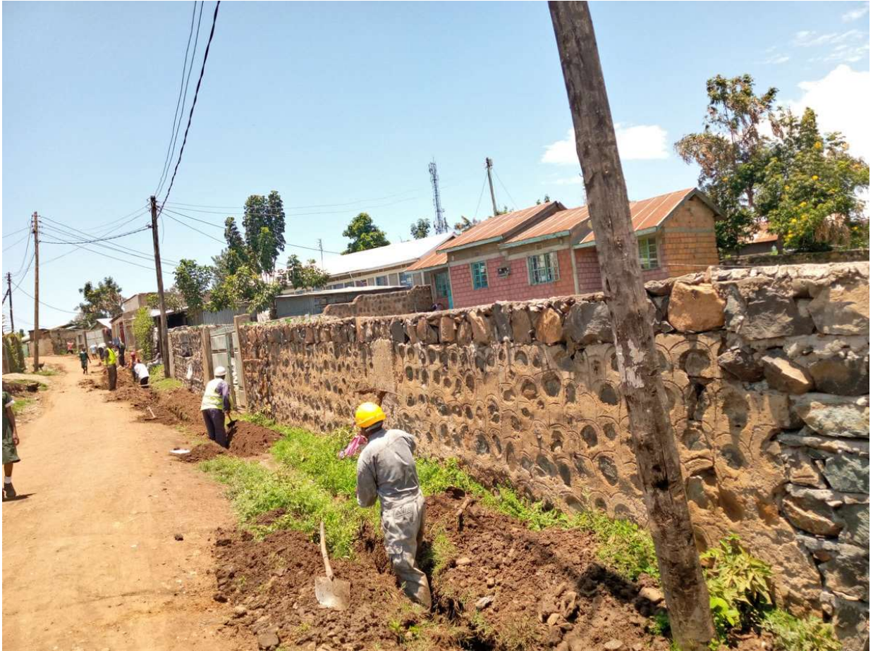
Installation of Delegated Management Model Meters in Kisumu ( Source: Practical Action in East Africa)
