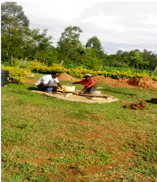
Photo2: Shallow well artisans excavating the well manually to remove sediments behind them
