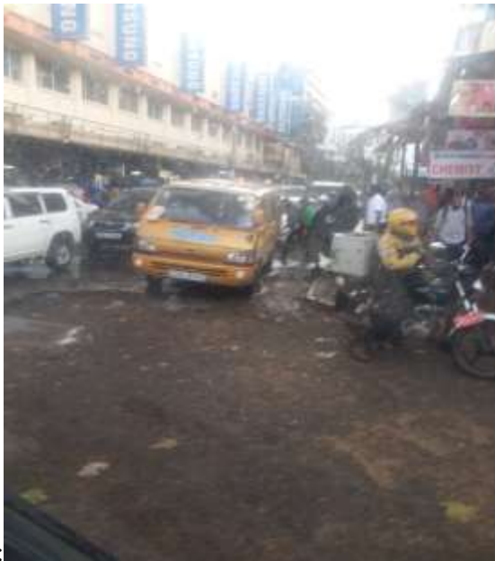
a. A large pothole at the junction of Tom Mboya Street and Mondlane Street.
