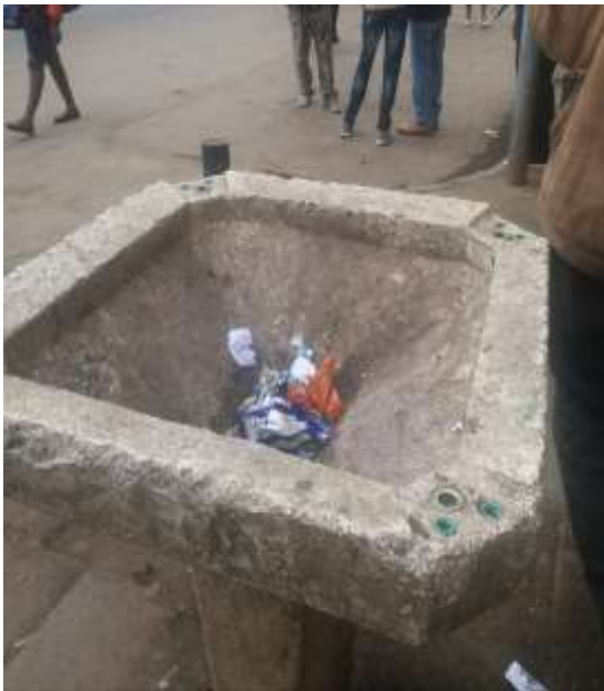
Plate 3.4: A faulty water point along Tom Mboya Street.
