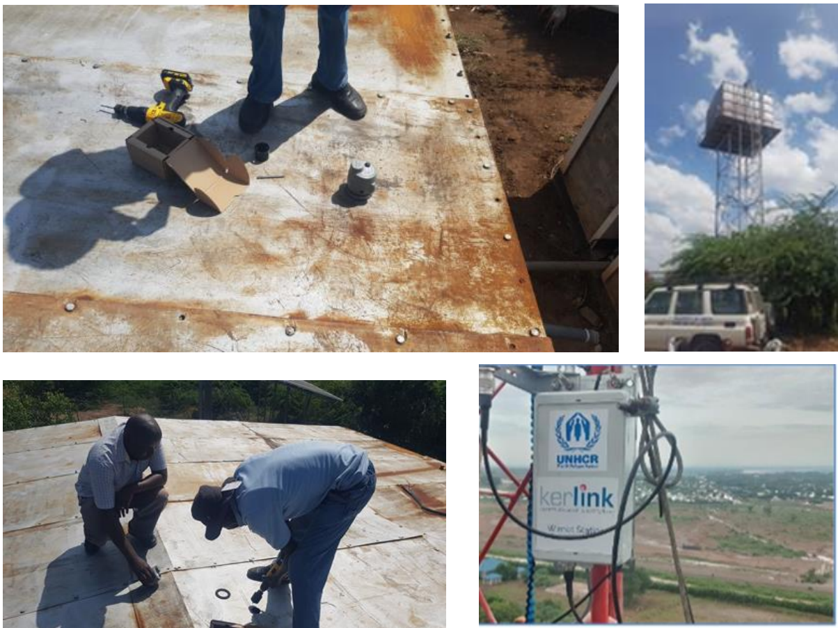
Figure 3.3 Installation of LoRaWAN Water level sensor
