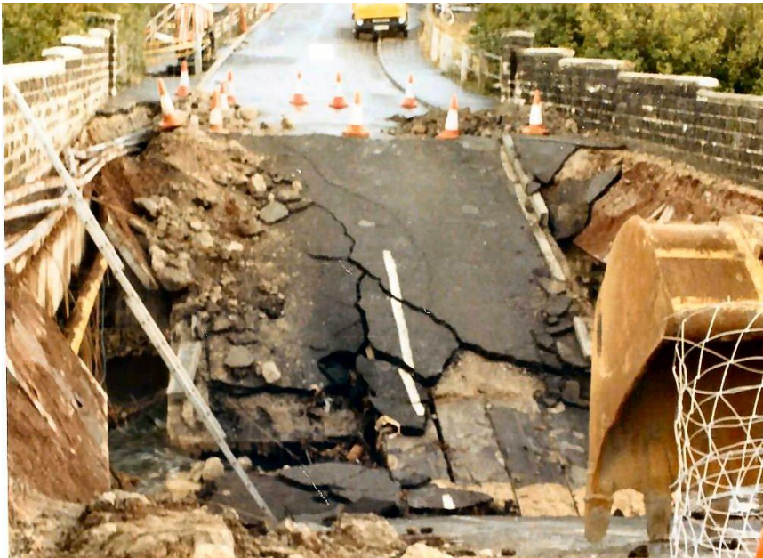
Figure 2.2: Collapsed Ynys-y-Gwas bridge [27]
