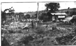
A general view of the alignment of the proposed Spillway which will be 500 feet long.
