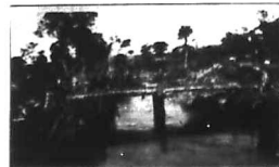
A temporary bridge over the back water erected for the purpose of conveying material which will be used in the construction of the Spillway.
