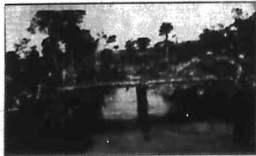
A temporary bridge over the back water erected for the purpose of conveying material which will be used in the construction of the Spillway.
