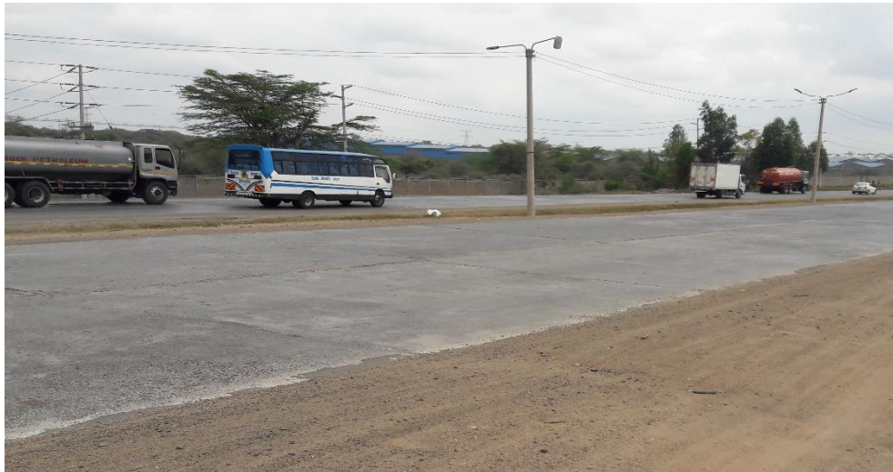
Plate 4-7: Section replaced with a rigid pavement due to repeated shoving.
