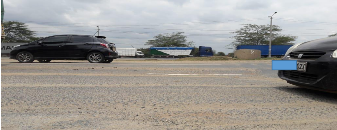
Plate 4-2: Excessive rutting on pavement surfacing
