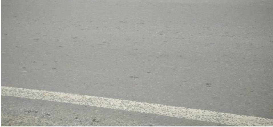
Plate 4-6: Bleeding of the asphaltic binder
