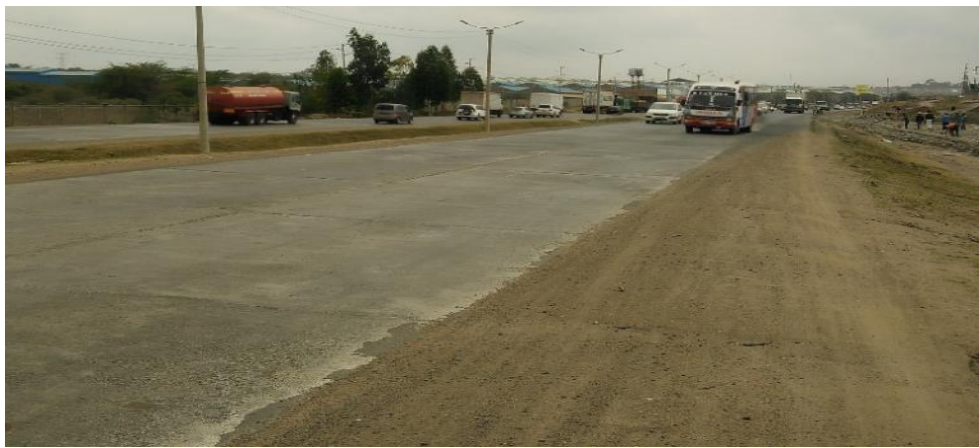
Plate 4-1: Longitudinal and transverse cracking of pavement surface
