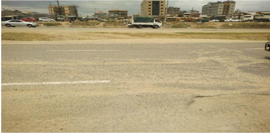
Plate 4-4: Corrugations on the pavement surface
