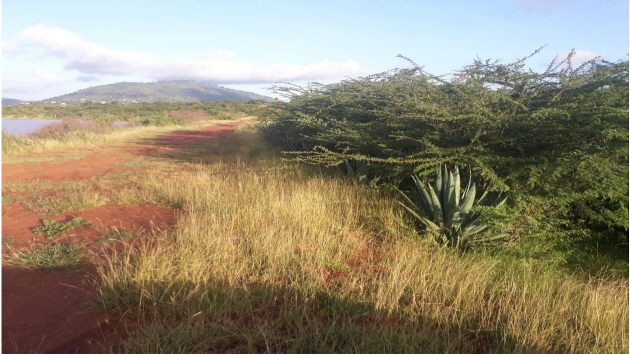
Figure 4.15: Trees Growing on Maruba Dam Embankment
