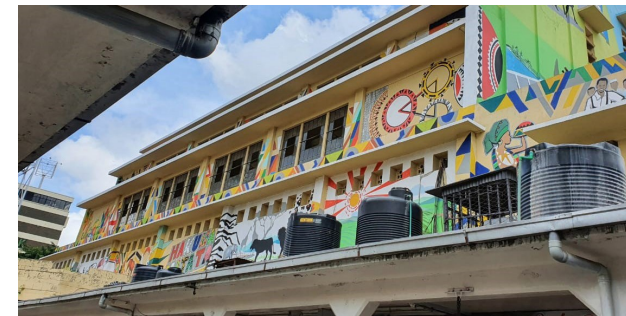
Fig2.10. Horizontal sun shading devices at City Market, Nairobi. Type A according to fig 2.8. Source: Author
