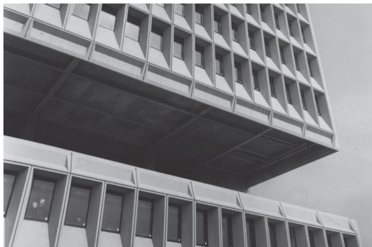
Fig 2.54. Scoring lines on concrete in Michael Breuer's molded facade.
