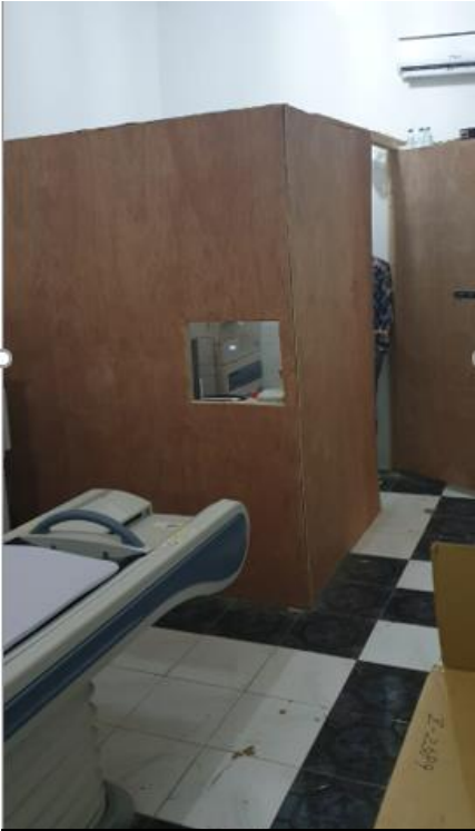
Image 5: Control room located inside CT room with uncovered roof
