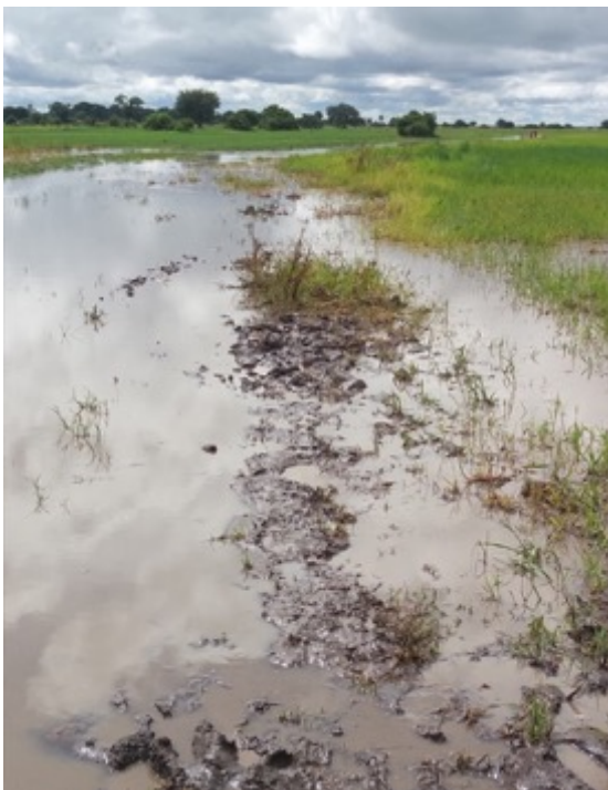
Picture 6.3: Flooded road
