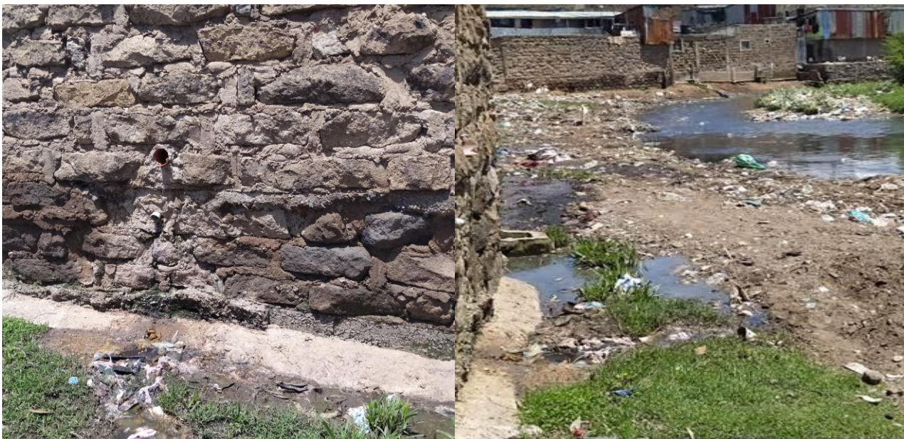
Plate 23 : Sewer outlet discharging directly into Ngong River
