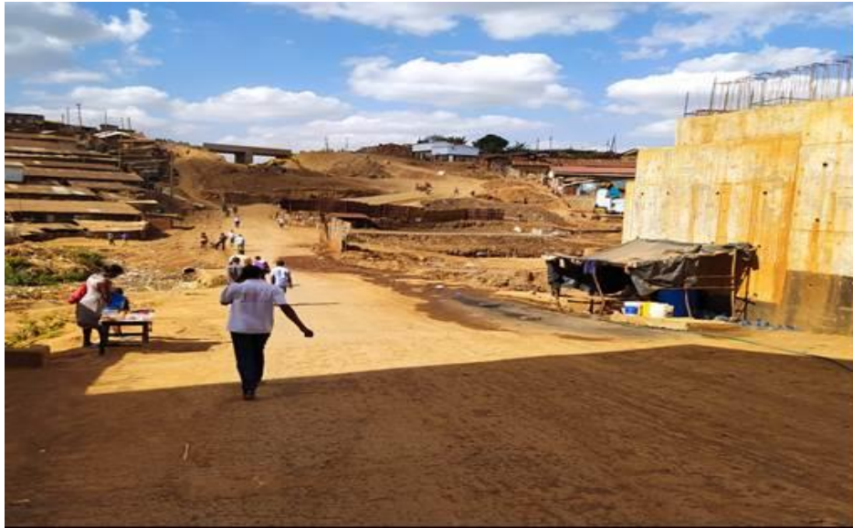
Plate 6 : Ongoing Road construction near Ngong River at Lindi Mosque, Kibera Source: Field data (2021)
