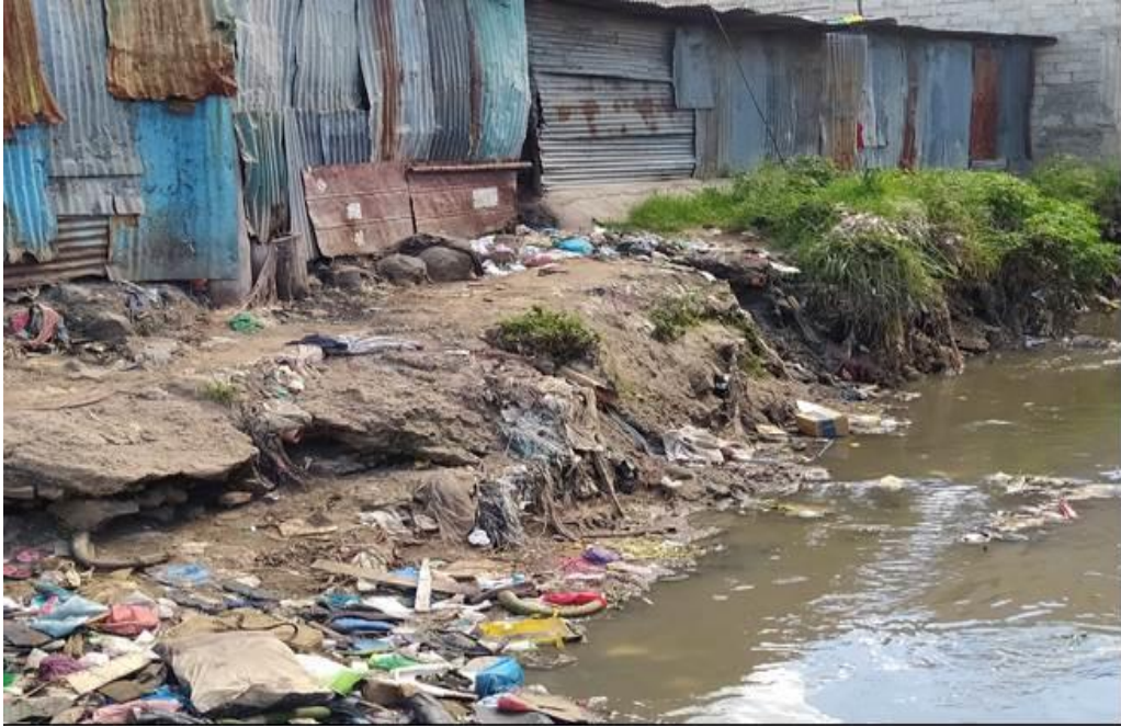
Plate 11 : Direct sewer discharge into Ngong River by informal settlements at Mukuru Kayaba (wet season) Source: Field data (2021)
