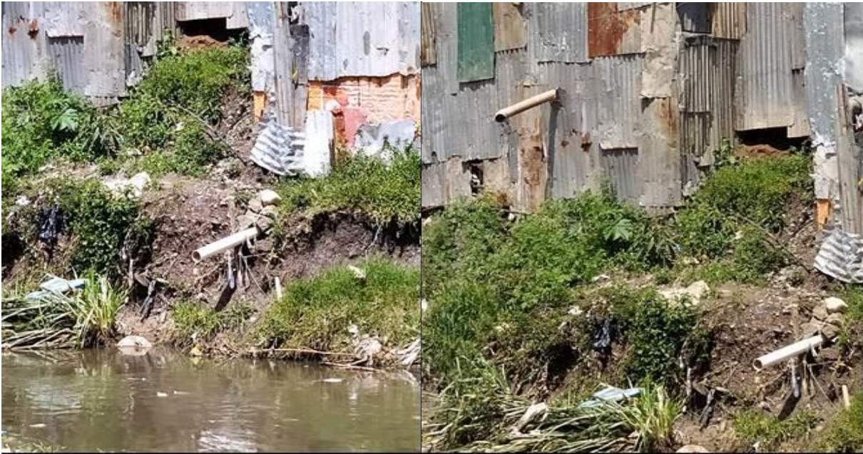
Plate 18 : Sewer pipes from the Mukuru Kwa Reuben Informal settlements along Enterprise Road discharging Sewage directly into Ngong River Source: Field data (2021)
