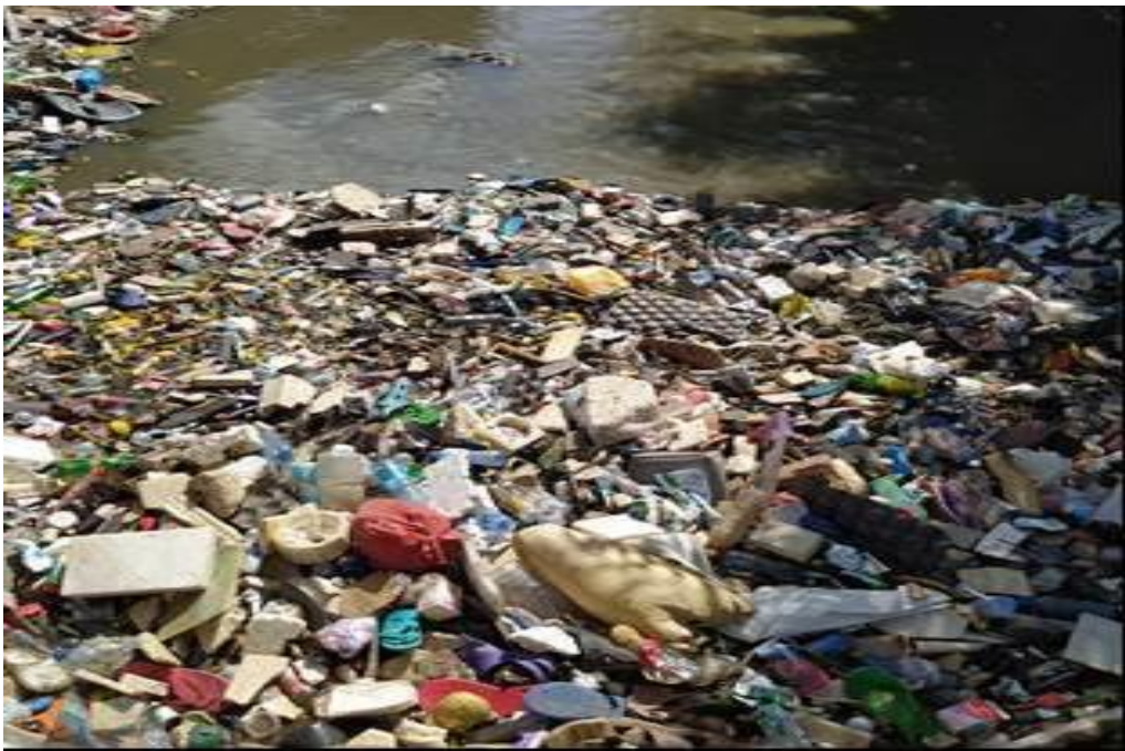
Plate 12: Solid waste clogging Ngong River Channel at Mukuru Kayaba Bridge (wet season) Source: Field data (2021)
