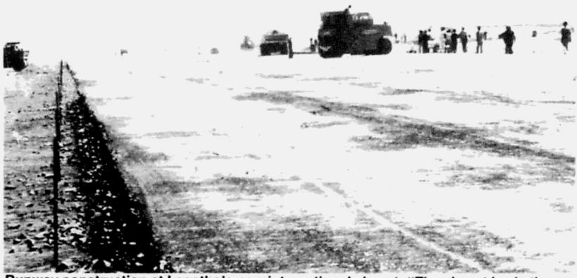
Runway construction at Lesotho's new international airport: "The airport is six times more costly than any other project Lesotho has ever seen"
