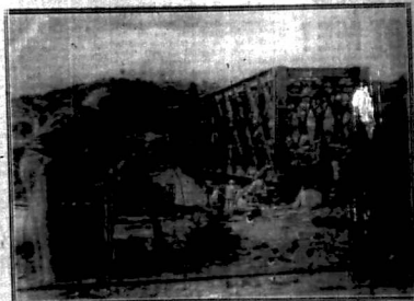
The new bridge, which was built in just over five weeks entirely from material salvaged from the old bridge, by 8 officers and 5 other ranks, entailed a four mile diversion which permitted the new bridge to be built at a level of 60 feet instead of the old high level of 202 feet. (Official War Office Photograph)
