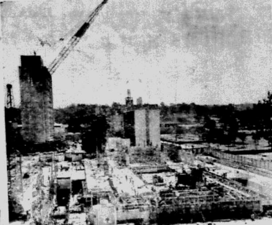
View of the construction site for the new berths at Kilindini docked yesterday. The new berths will be part of the port's expansion programme.
