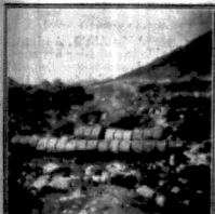
Wrecked culverts after a thunderstorm on the Nairobi-Magadi road.
