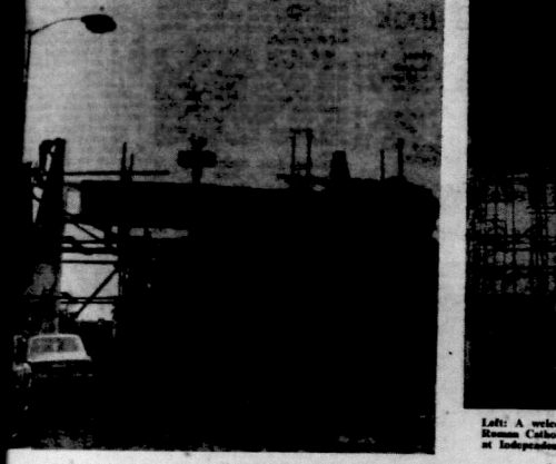
Left: A welcome arch for the Pope, under construction, at the approach to Rubaga Roman Catholic Cathedral. Above: A massive 17-ft. crucifix is placed in position at Independence Park, Kampala, on the platform on which the Pope will consecrate 12 Bishops on Friday.
