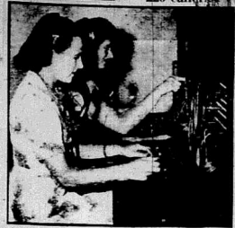
Brought into operation in the E.A.R. and M. Headquarters building, Nairobi, this week is this telephone exchange, with 20 double lines and the departmental lines. It will be capable of extension to 800-line capacity at short notice.
