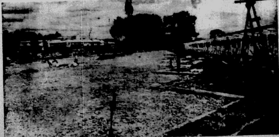
Work is well in hand at the site of Nairobi's new country bus station off Lamicho Road, where bus stands and paving are already in evidence and the ground is being staked.
