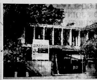
Work is progressing on the £200,000 Town Hall extension in Mombasa. Commencing in 1968, the new wing will house the departments of the Town Clerk, the Town Engineer and the Municipal Engineer. It is expected to be finished early next year.
