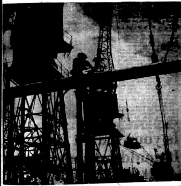
Workers of the Steel Construction and Painting Engineering Co., who installed and maintain the bulk molasses delivery pipe circulating the pipes on from the cliff top at Shimani in the region of the port.
