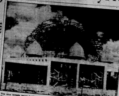
The new temple being built in the Sri Guru Singh Sabha in Jaipur, India, is to be nearly 90 feet high, cost £250,000 and will seat up to 5,000 people. The structure will be of granite masonry in yellow and red.
