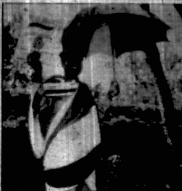
Work is not only on the pier but also on the pier's pier to land ships. The pier was made light of the rain of Wednesday yesterday.
