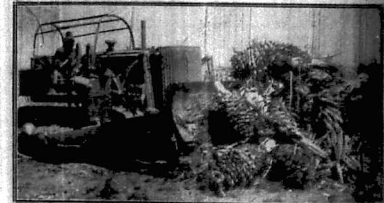
Silt reclamation work. Bull-dozing with a road-builder. (Photo: L. A. R. Powell)
