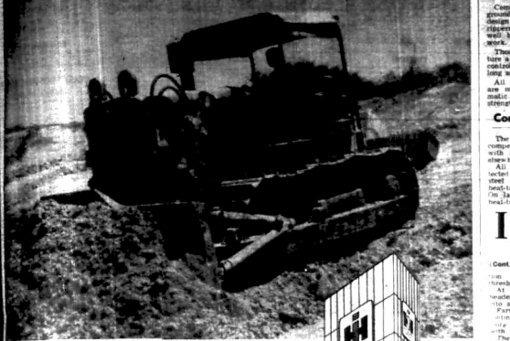
An International Series 20 Crawler tractor equipped with bulldozer blade and a ripper, as used in an East African rural quarry.
