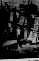
Self-help workers busy on the construction of a health centre at Mbaraka in the South Nyanza area.
