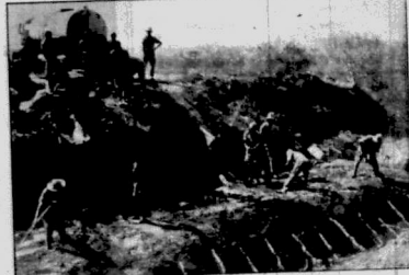
The job has been done on a good scale. The road is now open to traffic.
