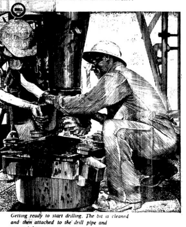
Getting ready to start drilling. The bit is cleaned and then attached to the drill pipe and screwed fast.
