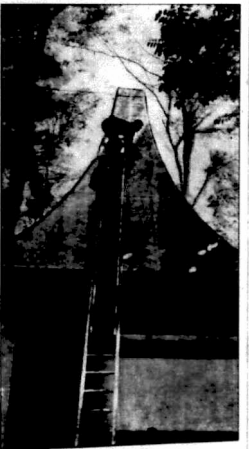
Above: Two workers found it a tough job putting the final polish on this copper-covered turret on one stand.
