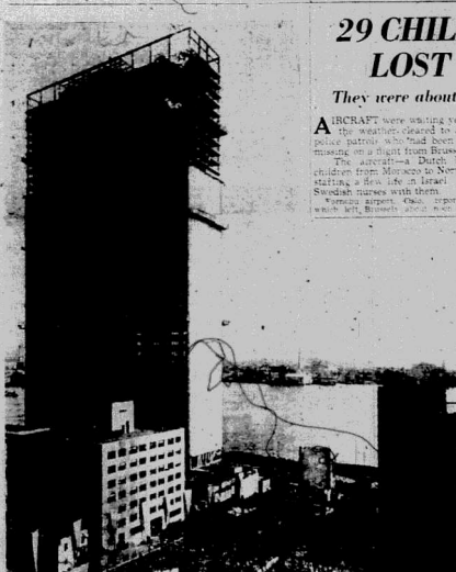
The 31 ton crane of the United Nations Secretariat Building was set on place during a special outdoor session of the United Nations General Assembly held at the site of the permanent headquarters of the organization in New York. President Truman, the Secretary of State, and other officials were present.
