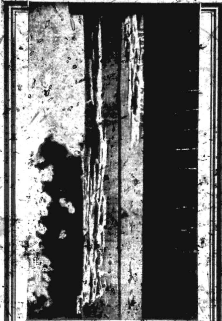
Due to lack of protection, the destruction caused by White Ants was so severe the structure had to be replaced in an incredibly short time.
